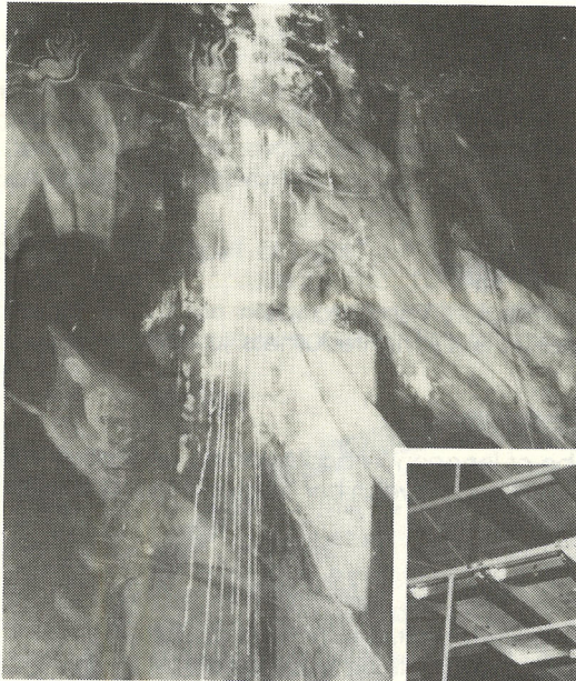
Moisture damage to "Spirit of Light" prior to restoration.
